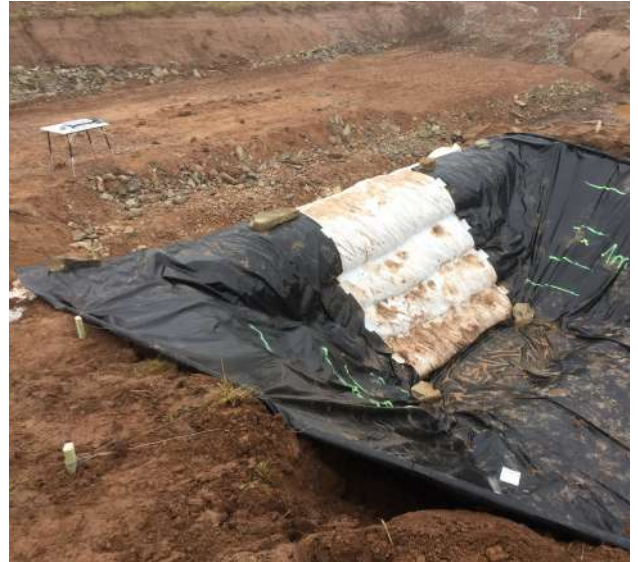
A geomembrane ground layer is used as a base for the pond.
