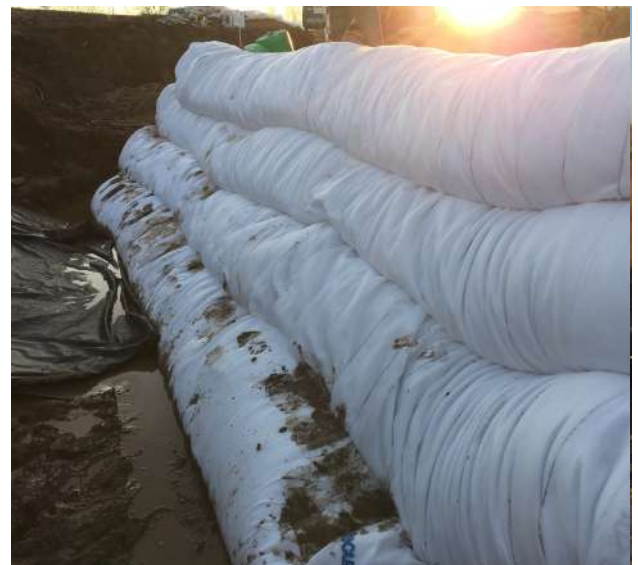
Several layer of topotube create a stable dam body. A steep ankle can be realized.
